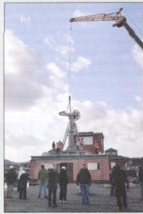
Picture courtesy of Daniel Lugo Photography Crews install a solar dish on the roof of the Flat Iron building in Bethlehem.
